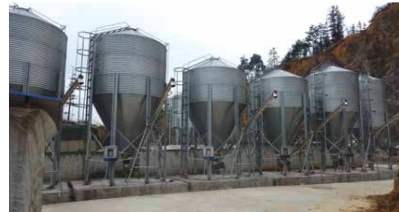
One production system Gillespie works with in China has changed from a bagged feed system to bulk deliveries, with trucks filling newly constructed bulk bins that are just inside the front gate.
